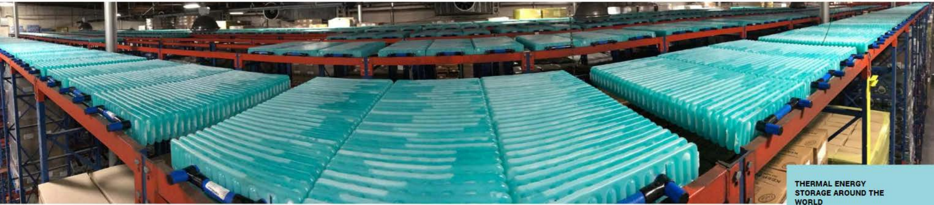
Viking Cold Solution's thermal storage cells at Dreisbach distribution center in Richmond, Calif.
